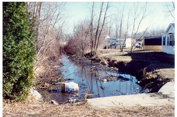
Poorly maintained urban drain with obstructions, eroding banks & human trash
