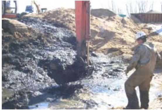
BELOW: Engineers have temporarily relocated the creek flow to allow access to the bottom sediments which were captured behind the dam. Specially trained haz-mat workers are shown removing the contaminated sediments from the creek bed. Clean replacement soils can be seen in the background.
