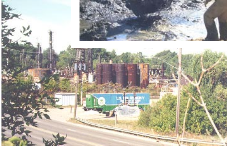
ABOVE: The EPA's mobile wastewater treatment plant is seen parked near Cork Street. Called "Springfield Belle," this trailer removes pollution from storm water runoff that is captured in sumps and lagoons during the cleanup.
